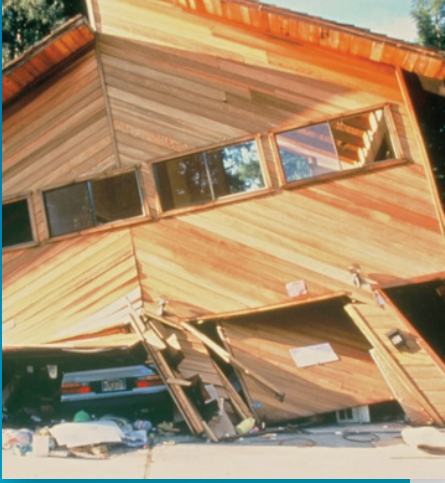
The walls around the garage door of this home were not strong enough to withstand the shaking of the 1989 Loma Prieta Earthquake.
