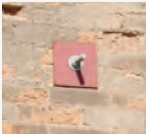
A steel plate with anchor bolts.
